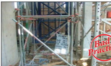
POOR ACCESS TO THE CRANE MAST
