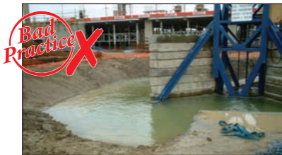
EXAMPLE OF A FLOODED TOWER FOUNDATION
