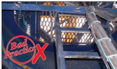
RESTRICTION OF LADDER WIDTH BY CABLES
